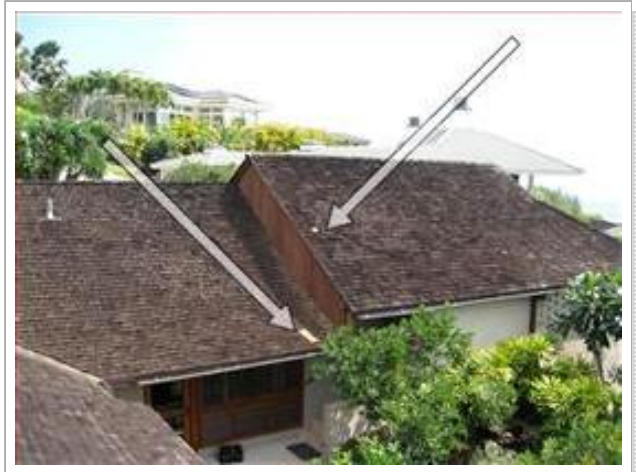
Missing shingles noted on various areas of roof. Repair/replace as needed.
