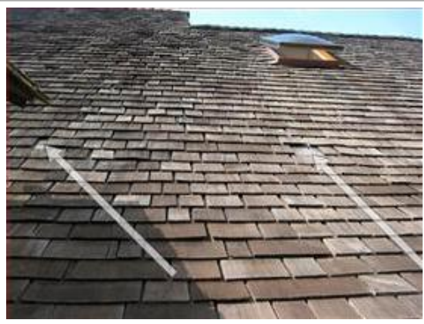
Missing shingles noted on various areas of roof. Repair/replace as needed.
